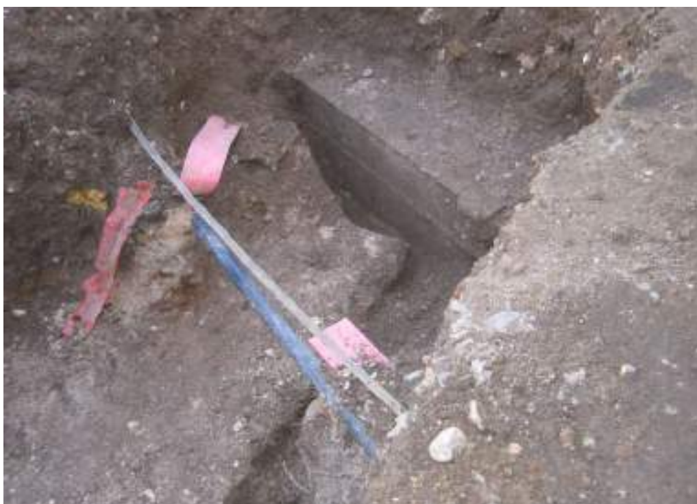
Sl. 10 Instalacije na uništenom spoju jugoistočnog i jugozapadnog zida Fig. 10 Installation on the destroyed junction of the south-east and south-west walls
